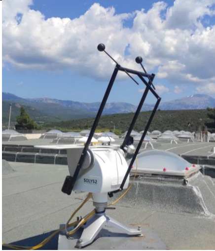
Figure 1: Instrumentation installed at Psachna, Evia.
